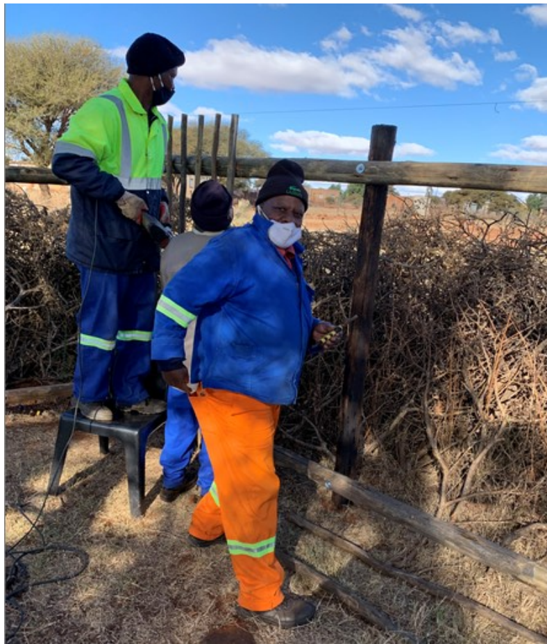
The second handyman in the project was Raneo Gaoboihe who was operating a drilling machine a, while Raditsheke Diphae was one of the foreman for the day.by the way each day was having its own foreman depending on the task/work at hand and Kalayakgosi and Sekgotlane were also very skillfull in the project.
